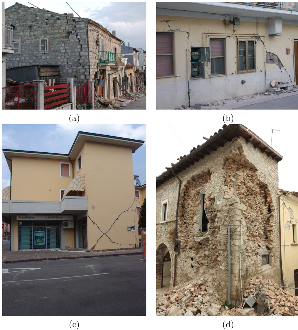
Fig. 1. Illustration of various unannotated images included in the employed training dataset. (a,b) City of San Giuliano di Puglia, Molise earthquake: (a) vertical crack causing the separation of two orthogonal masonry walls in a two-story building; (b) combination of horizontal, vertical, and diagonal cracks in the masonry portion (right side) of a mixed reinforced concrete–masonry structure. (c) City of Novi di Modena, Emilia–Romagna earthquake: X-shaped crack on the masonry wall of the right-hand portion of a building constructed in masonry, adjacent to an undamaged section built in reinforced concrete (left side). (d) City of Preci (Perugia), Norcia earthquake: spalling at the intersection of two orthogonal double-leaf masonry walls.
