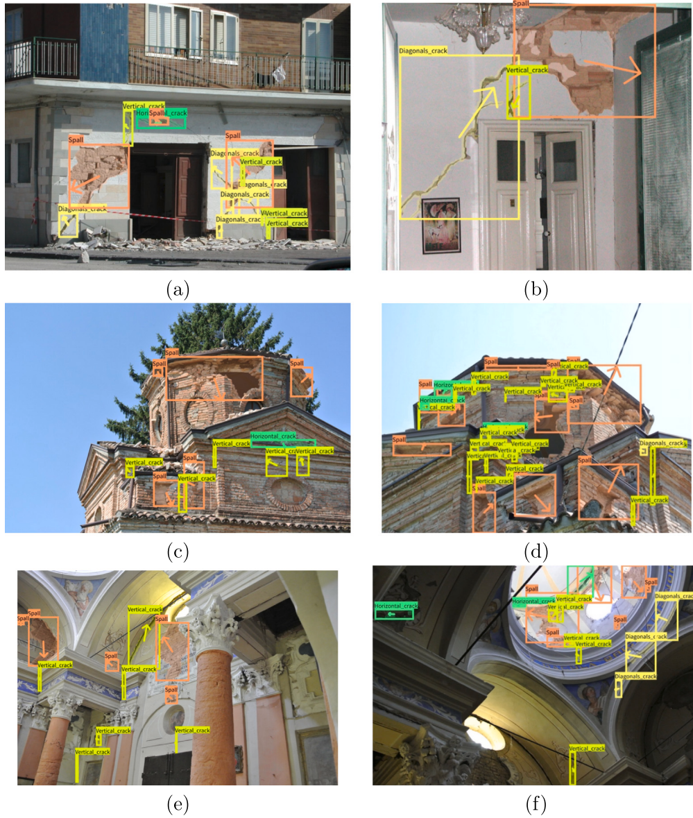
Fig. 7. Test phase: detection of damage in the images shown in Fig. 3.
