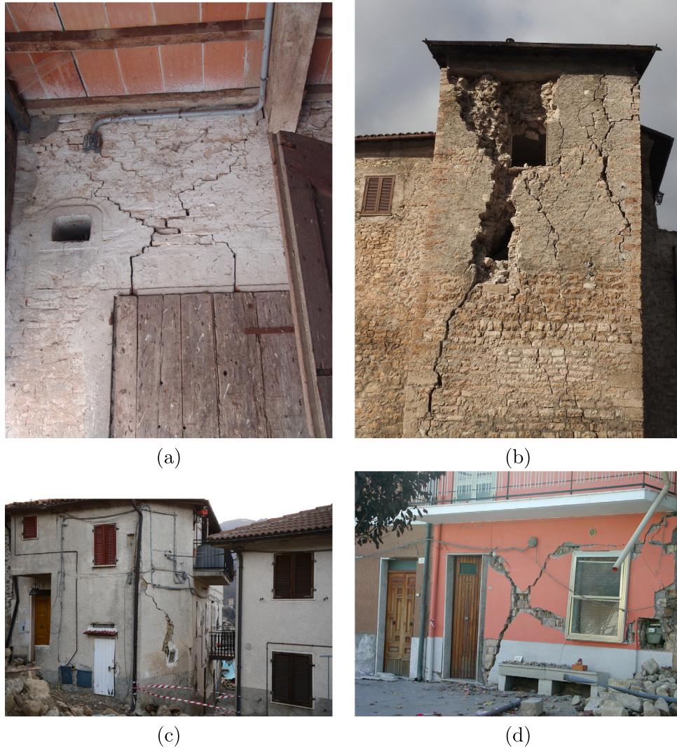
Fig. 2. Illustration of selected images contained in the validation dataset prior to annotation. (a) Crack damage inside a building struck by the 2012 Emilia–Romagna earthquake, visible above an opening lacking a reinforcing lintel; (b) Detection of masonry spalling on the external wall surface and cracking in a section of the city walls of Norcia, damaged by the 2016 earthquake, built with rubble-filled masonry; (c,d) Detection of shear cracking damage in two buildings in the city of San Giuliano di Puglia, struck by the Molise earthquake.
