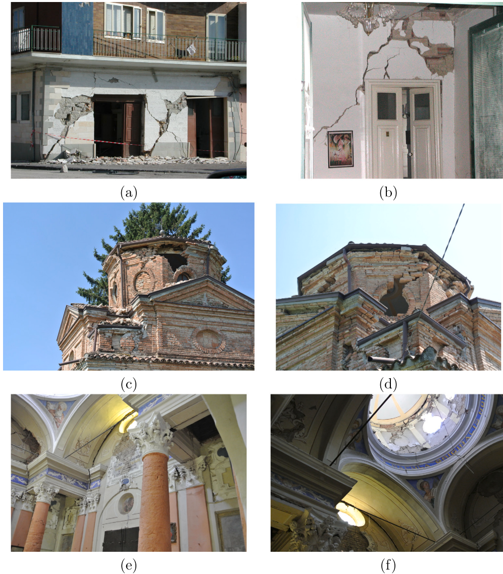
Fig. 3. Illustration of selected images included in the test dataset before the application of the CNN damage-detection procedure. (a,b) Shear damage on the ground floor (a) and in the interior (b) of buildings located in the city of San Giuliano di Puglia, affected by the 2002 Molise earthquake; (c–f) Cracking and spalling damage observed on both the exterior and interior of the Gasparini Casari Chapel, located in the Province of Modena and affected by the Emilia–Romagna earthquake.
