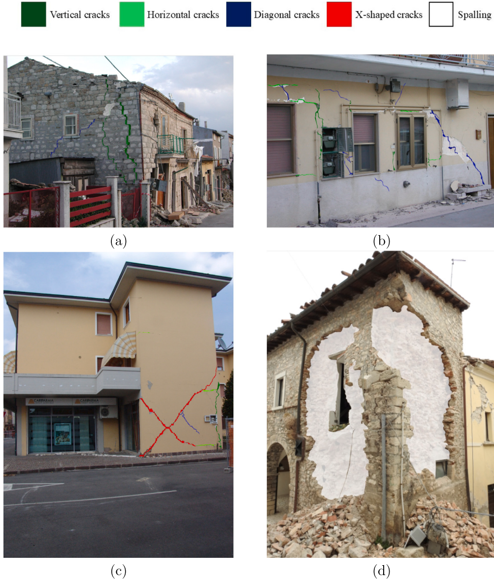
Fig. 5. Training phase: annotation of the images shown in Fig. 1. In this and the following figures, the defined damage classes include vertical, horizontal, diagonal, and X-shaped cracks, as well as masonry spalling, represented by the color codes displayed at the top of the figure.
